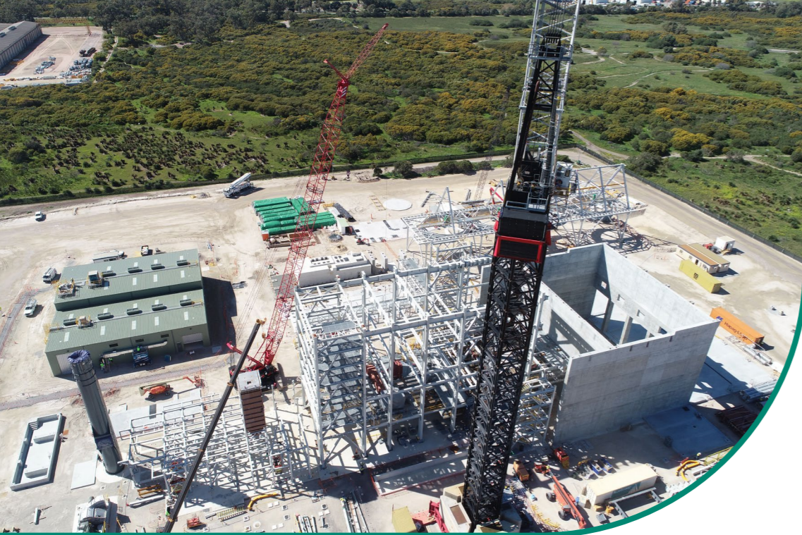
Image: East Rockingham Waste to Energy (ERWTE) – Rockingham WA.
